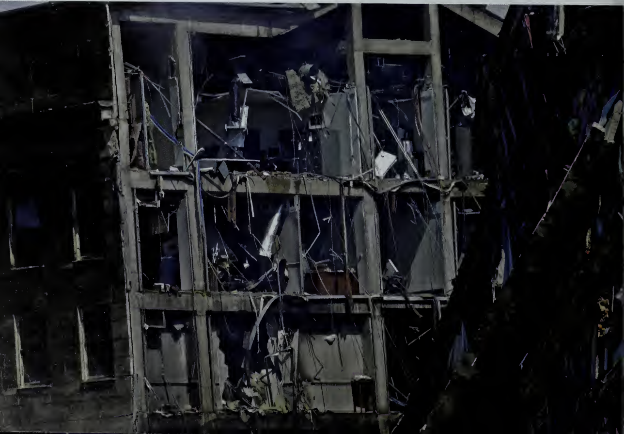
Damaged interior offices sheared open by the collapse of the E Ring.
